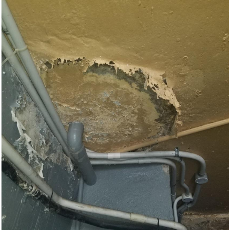
Image 44: Showing Minor Operations Soffit showing peeling.
