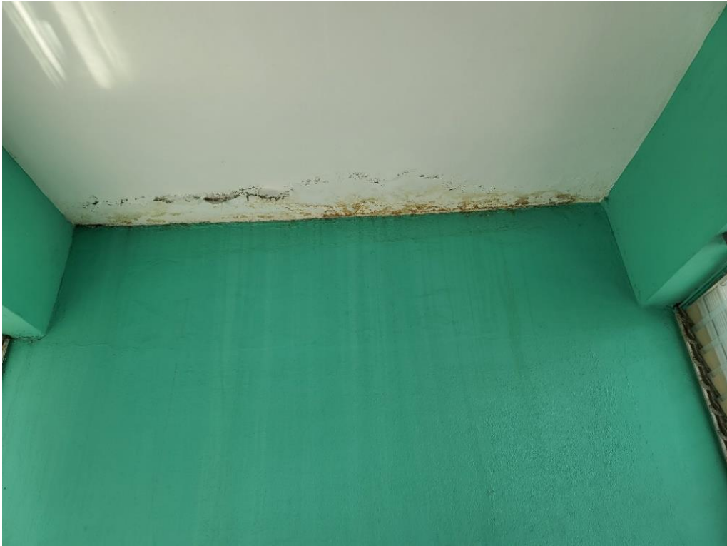
Image 72: Showing Damaged Soffit at Labour Ward
