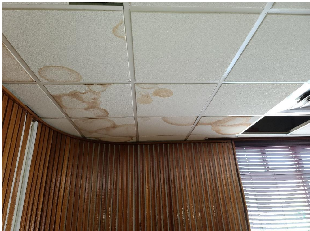
Image 63: Showing signs of leakage in Administration Building Ceiling
