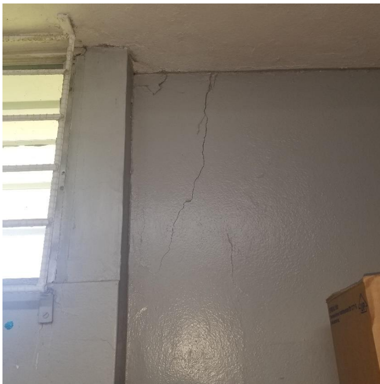
Image 55: Showing Crack in Wall at X-Ray
